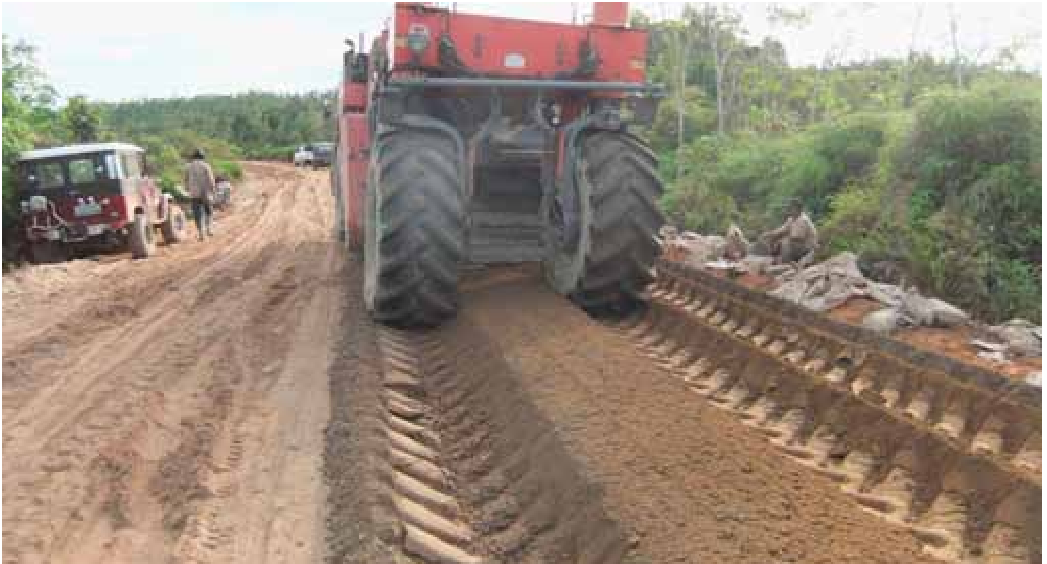
Milling of the cement-Novocrete® mixture up to a depth of 35 cm by adding water
