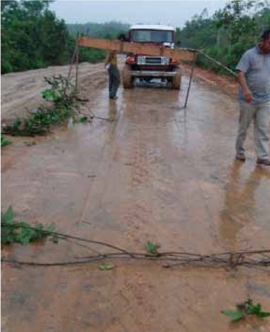
The finished road is irrigated several times and then blocked for the traffic
