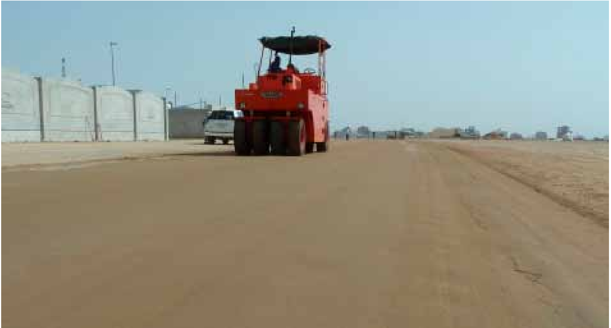
Final compaction with a rubber-tyred street roller to achieve a perfect surface of the area
