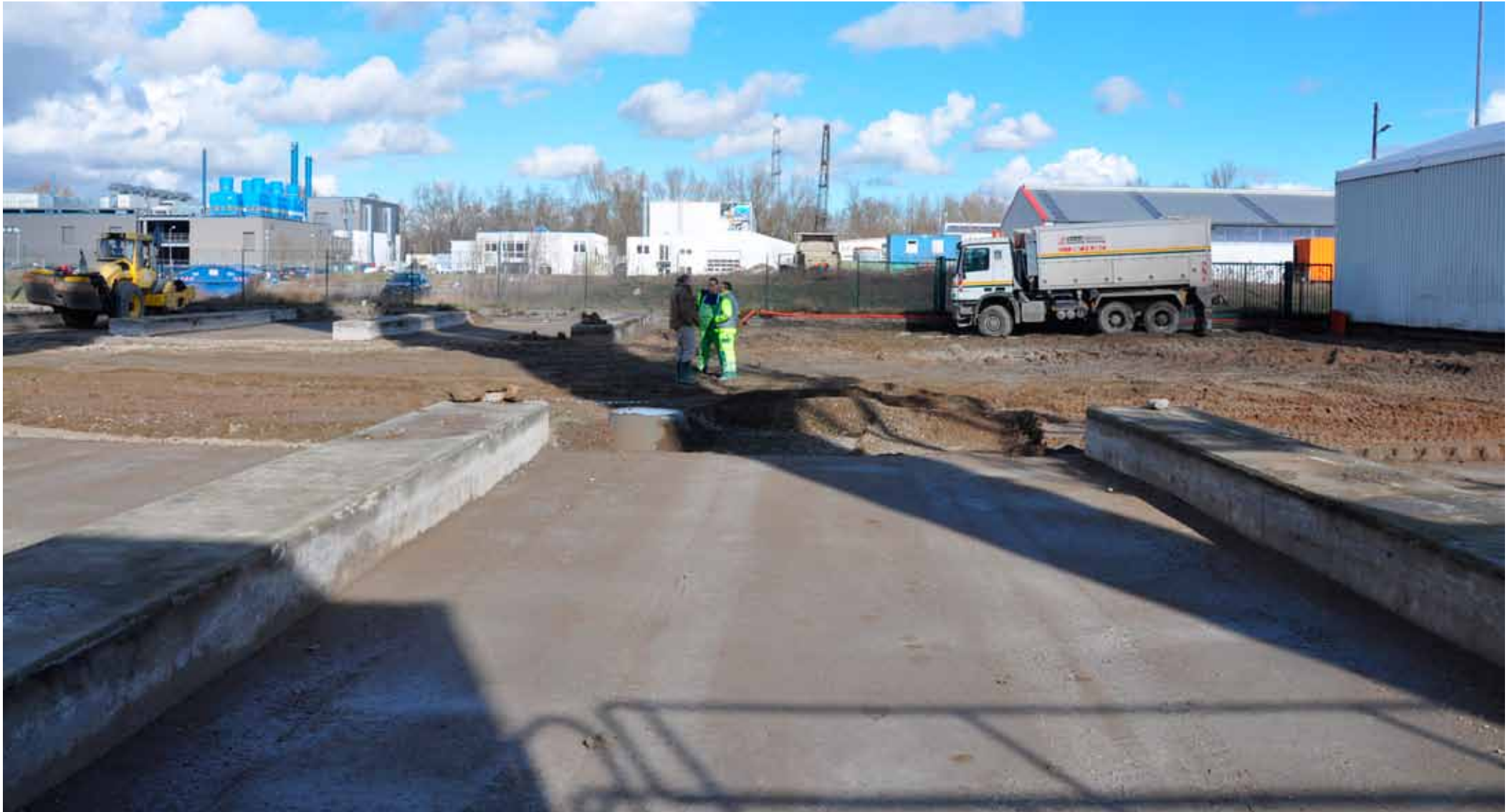
Stabilized area after one day - values in load bearing capacity > 300 \text{ MN/m}^2
