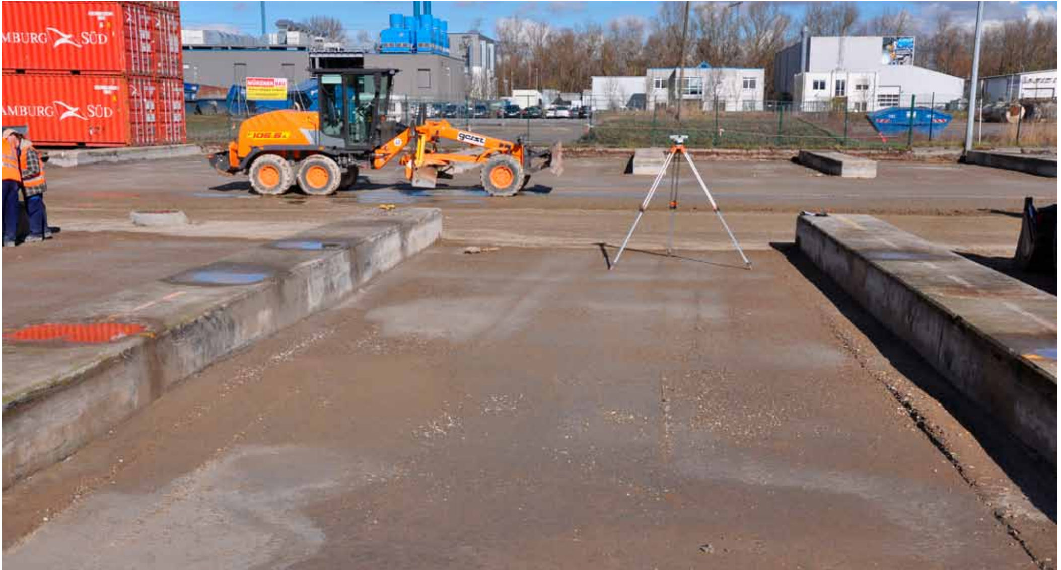
Stabilized area after one day - values in load bearing capacity > 300 \text{ MN/m}^2
