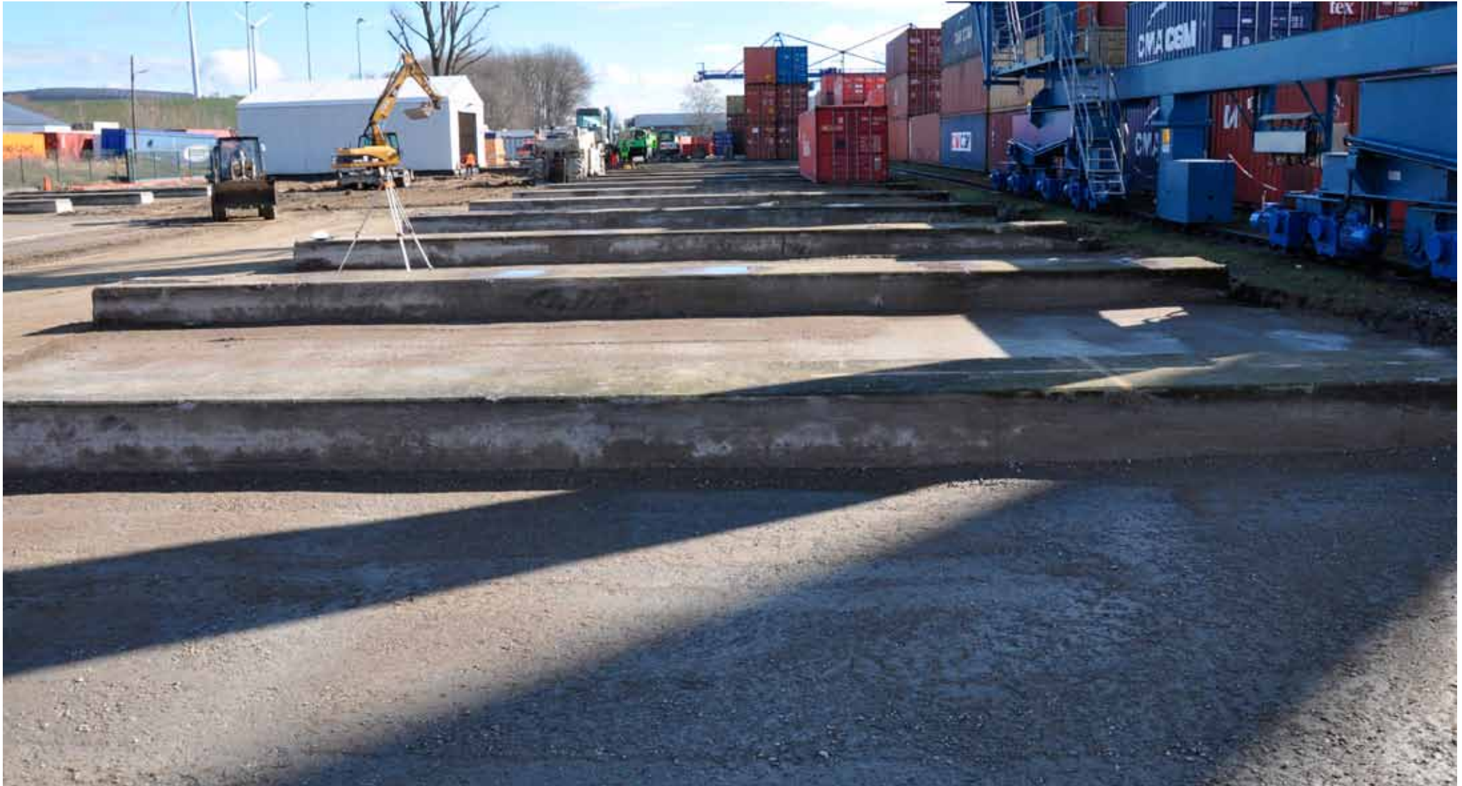
Stabilized area after one day - values in load bearing capacity > 300 \text{ MN/m}^2
