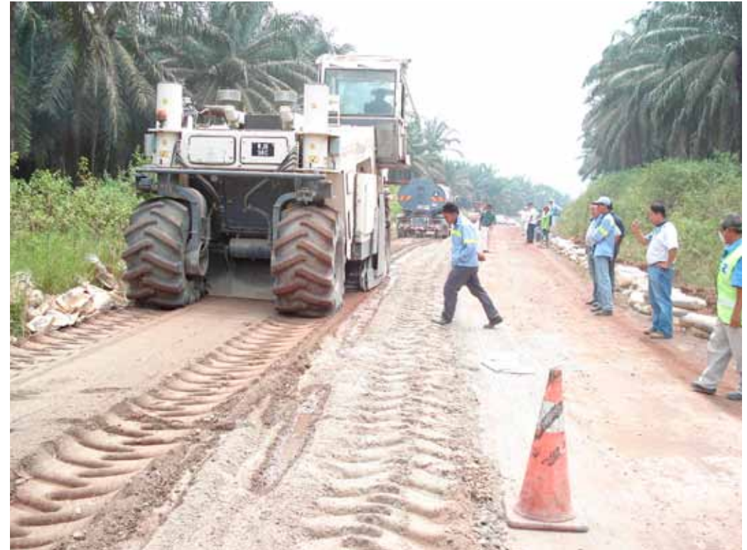
Fig 5: Incorporating the NovoCrete® ST cement mixture into the natural lateritic soil with a WR® 2500. Before, the mixture was irrigated by means of a road tanker driving ahead.
