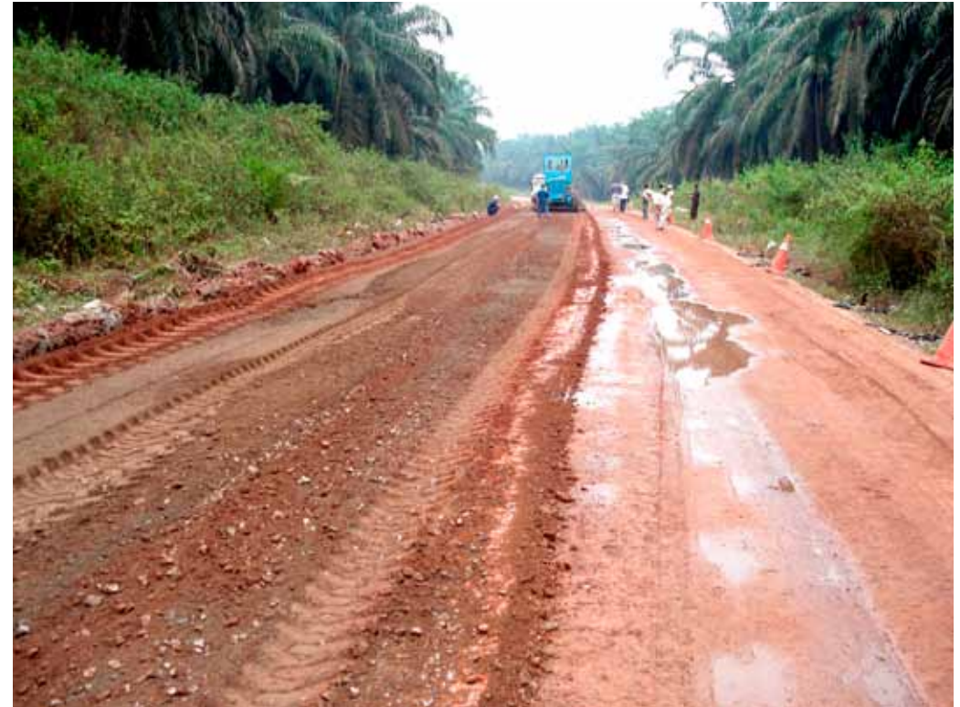
Fig 7: Forming the finish subgrade by means of a grader, while the right side of the road has already been compacted
